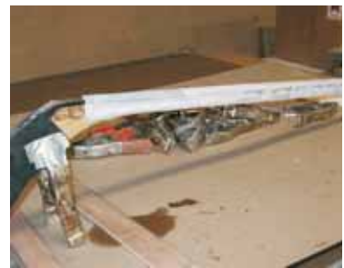
4. Apply a layer of fiberglass tape to the repair area with G/flex 650 for additional reinforcing.
